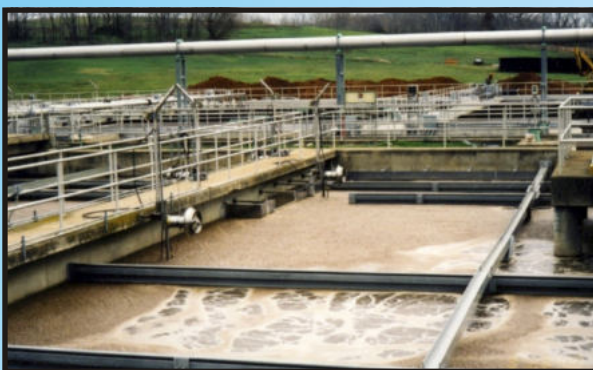
Effluent Treatment Plant
